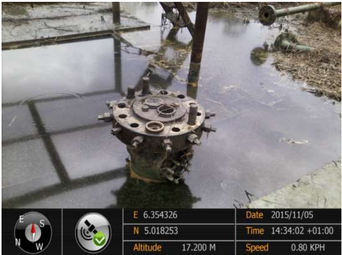
Close-up: No source of leak observed on Etelebou Well6T. Picture was taken during Joint Investigation of 5 th November 2015.
