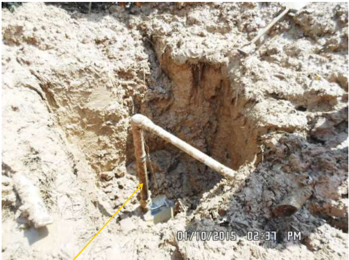
Close-up: Illegal fitting on 20" Kolocreek-Rumekpe Trans Niger Pipeline at Oda. Picture was taken during Joint Investigation of 1 st October 2015.
