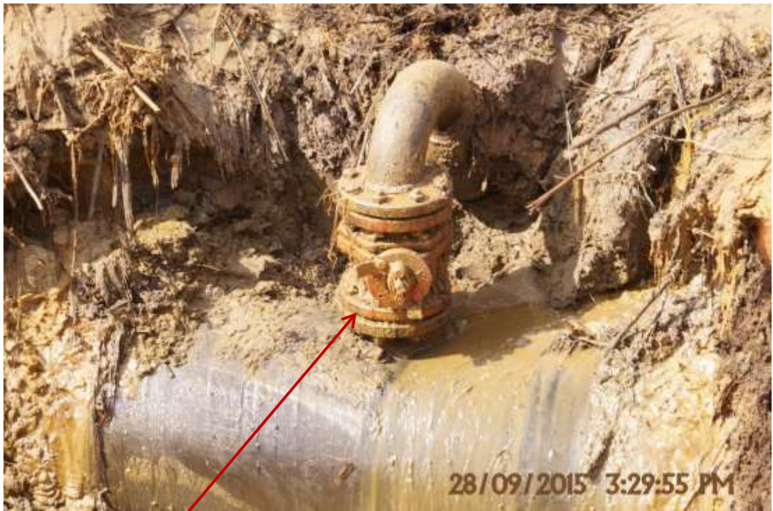
Close-up: Illegal fitting on 24" Trans Escravos Pipeline at Sokebolou. Picture was taken during Joint Investigation of 28 th September 2015.
