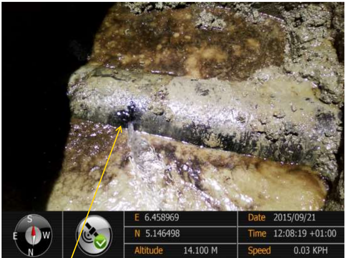
Close-up: Hacksaw cut on 14" Okordia-Rumuekpe Pipeline at Ikarama. Picture was taken during Joint Investigation of 21 st September 2015.
