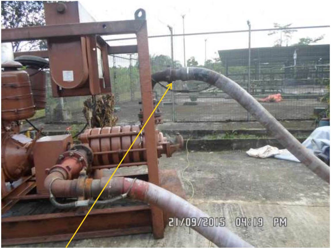
Close-up: Spill point on Etelebou Flowstation Manifold at Ogboloma. Picture was taken during Joint Investigation of 21 st September 2015.
