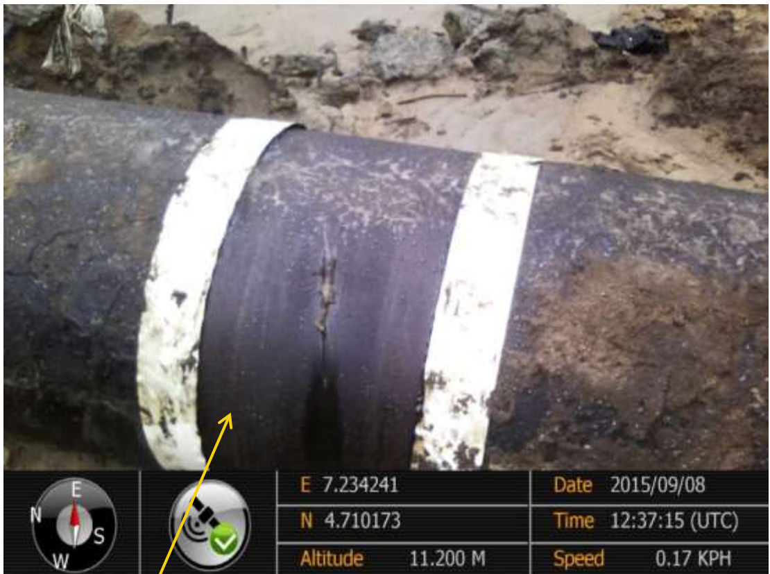
Close-up: Clamp illegally removed on 28" Nkpoku-Bomu Pipeline at Kporghor/Gio. Picture was taken during Joint Investigation of 8 th September 2015.
