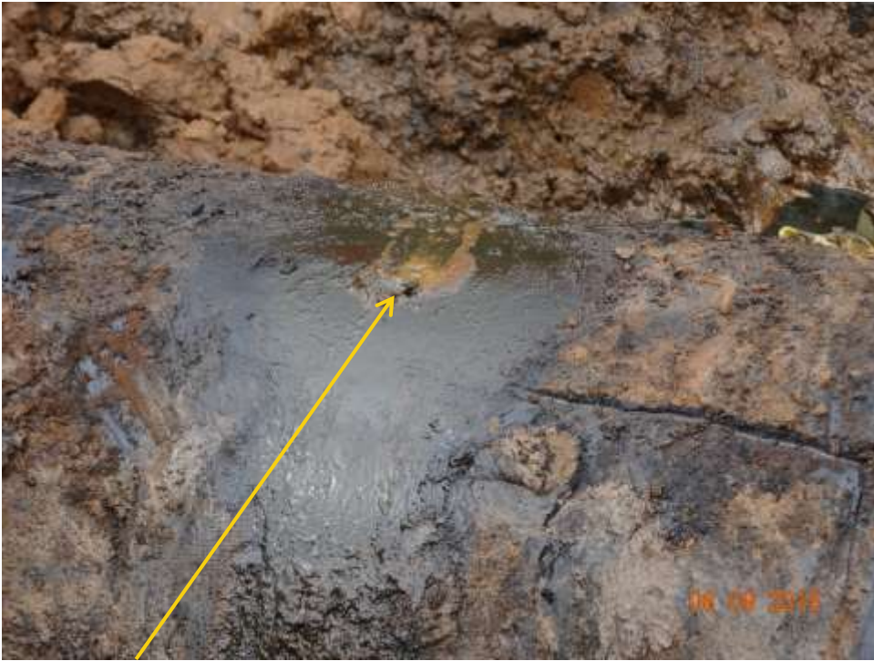
Close-up: Multiple drilled holes clustered together pictured after plugging on 28" Nkpoku-Bomu Pipeline at Norkpo. Picture was taken during Joint Investigation of 6 th September 2015.
