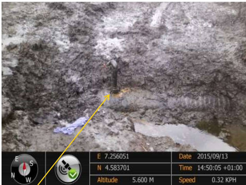
Close-up: Illegal fitting on 28" Bomu-Bonny Pipeline at Bodo West. Picture was taken during Joint Investigation of 13 th September 2015.
