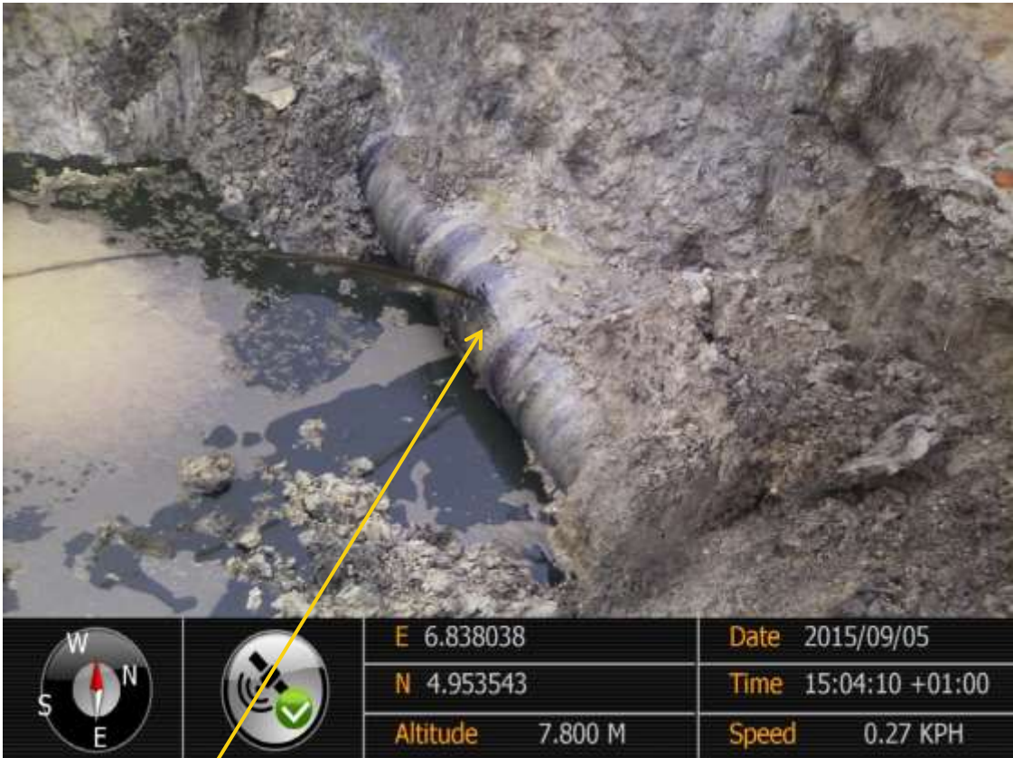
Close-up: Drilled hole on 20" Rumuekpe-Nkpoku Pipeline at Omuigwor/Ibaa. Picture was taken during Joint Investigation of 5 th September 2015.
