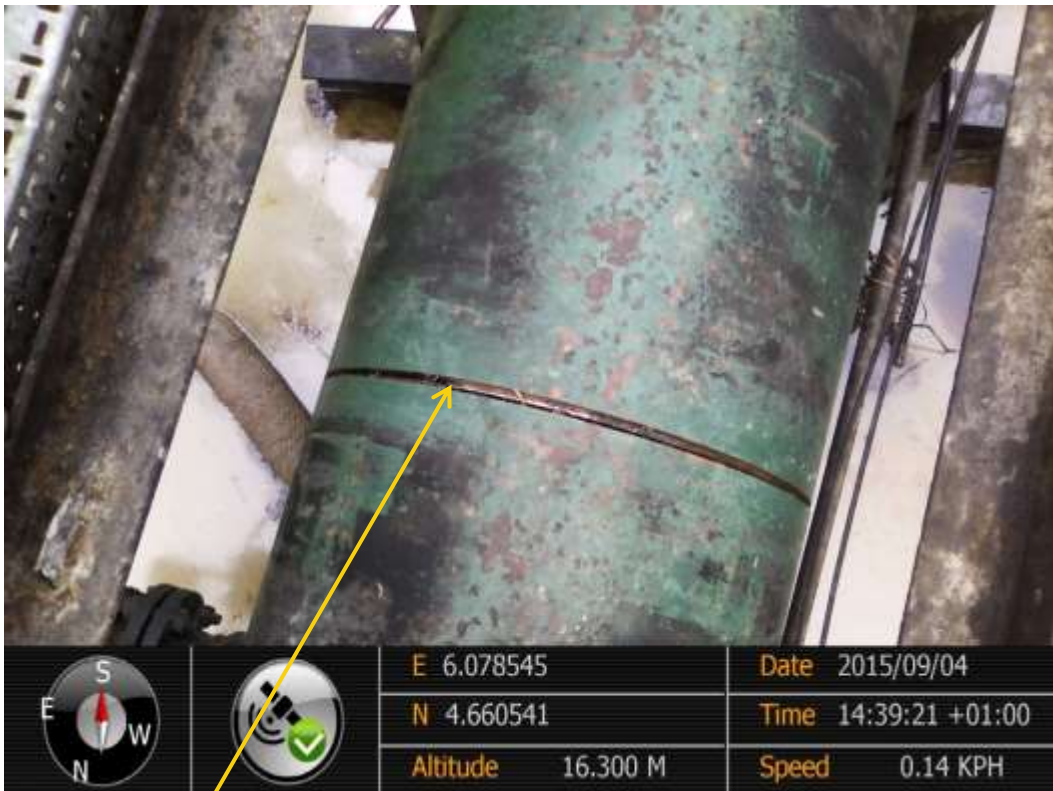
Close-up: Source of spill (backflow) during planned site works at Diebu Creek Flowstation 24" Flarehead Line at Peremabiri. Picture was taken during Joint Investigation of 4 th September 2015.
