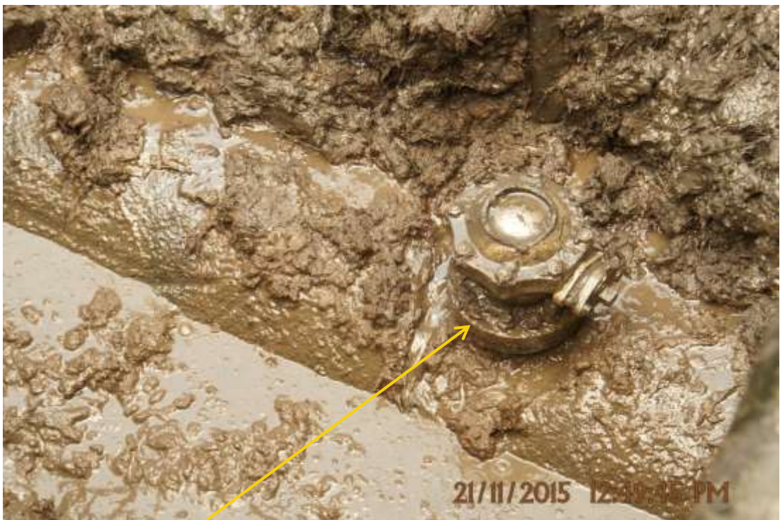
Close-up: Illegal fitting on 16" Tunu – Brass Creek Pipeline at Agbidiana. Picture was taken during Joint Investigation of 21 st November 2015.
