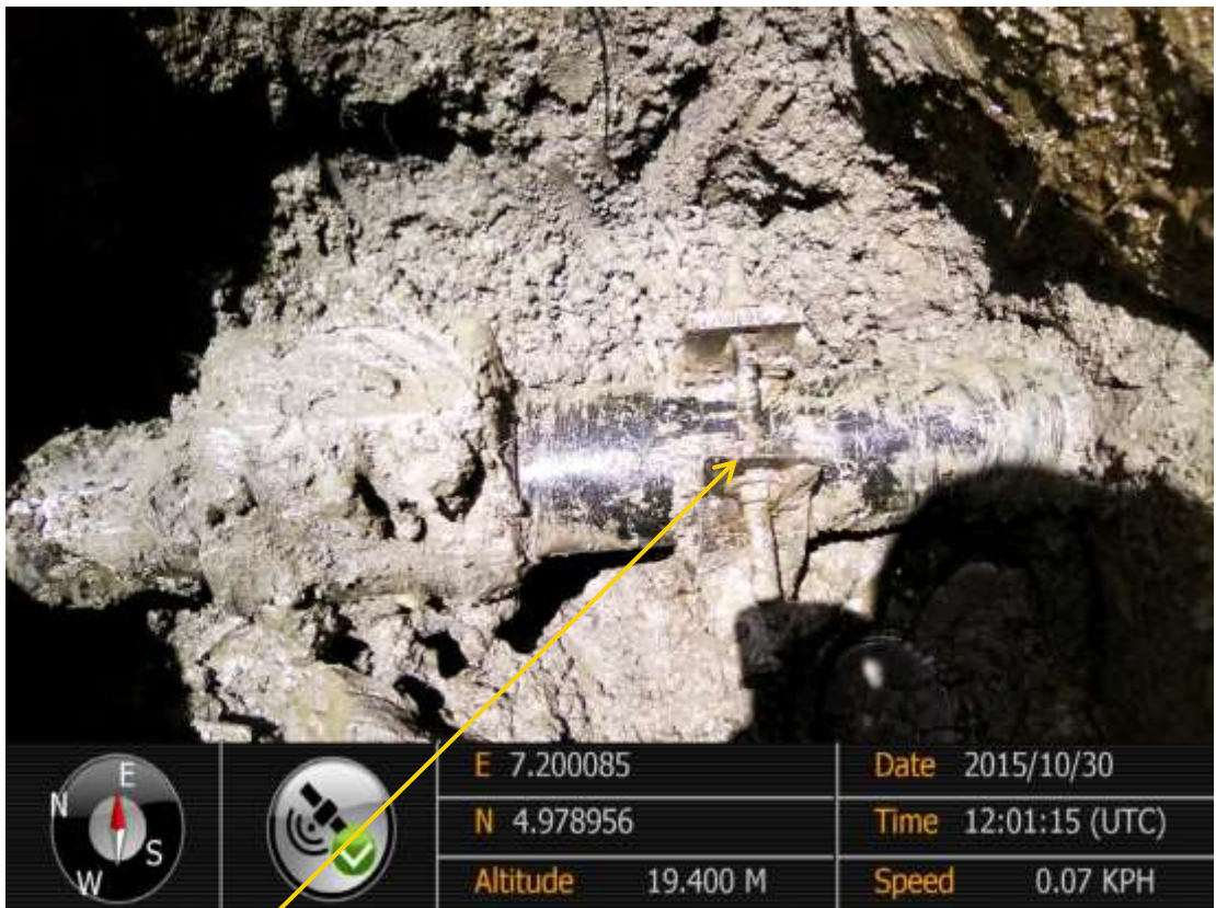
Close-up: Illegal fitting on Imo River Well 33L Flowline at Ipu West. Picture was taken during Joint Investigation of 30 th October 2015.
