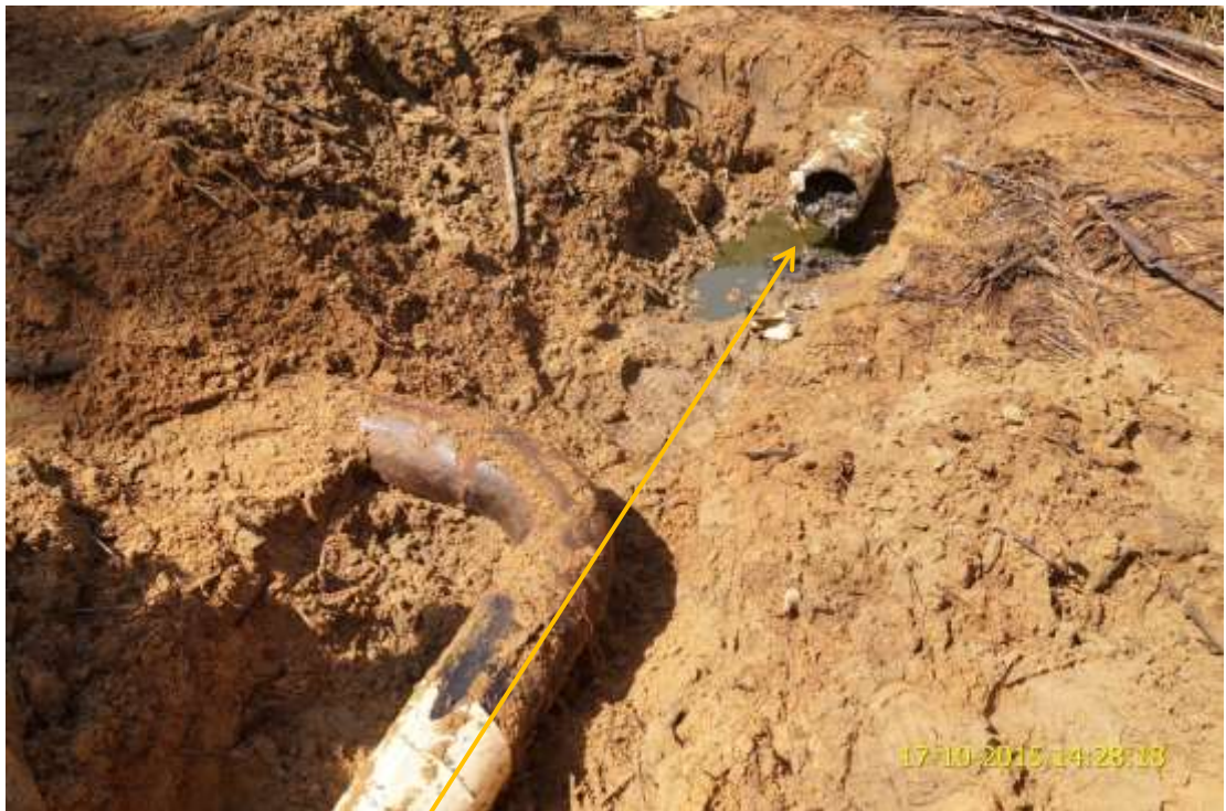
Close-up: Cut section of missing flowline on 6" Yokri Manifold1 Disused Flowline to Cluster 95 at Obotobo. Picture was taken during Joint Investigation of 17 th October 2015.
