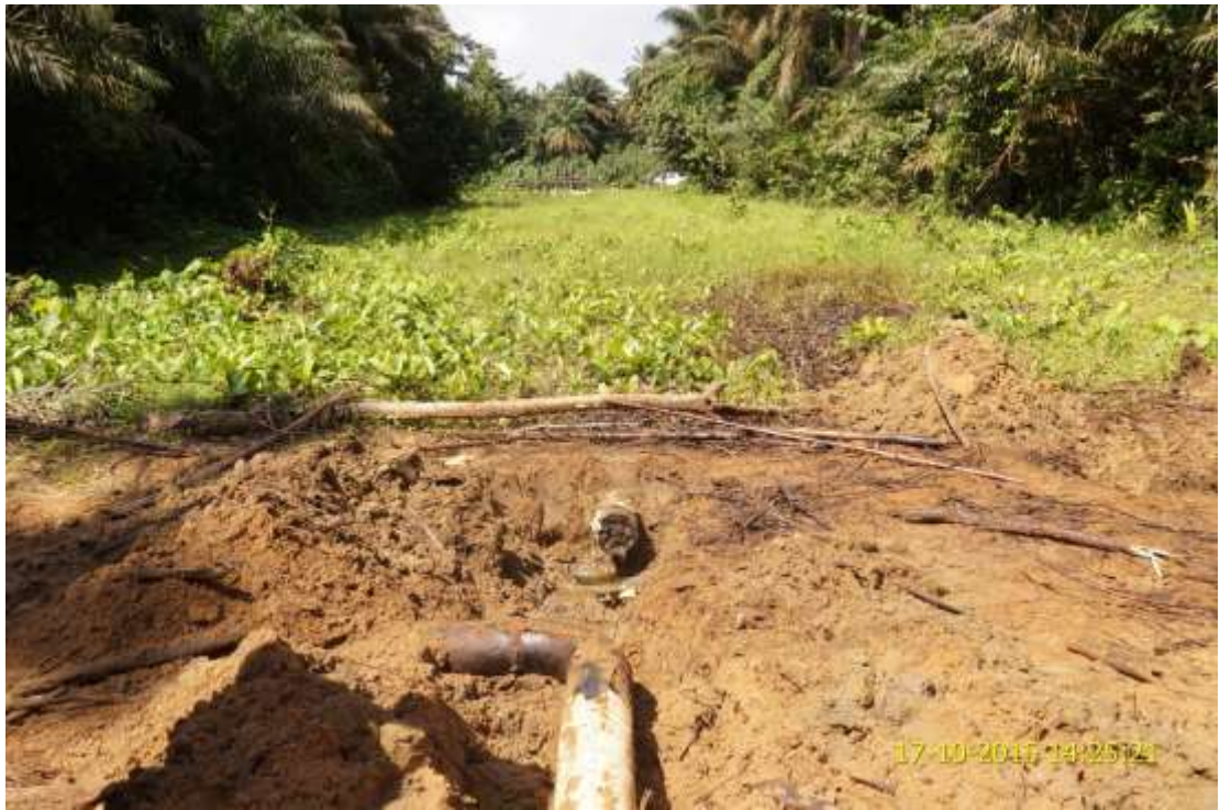
Overview: Part of spill impact on 6" Yokri Manifold1 Disused Flowline to Cluster 95 Right of Way at Obotobo. Picture was taken during Joint Investigation of 17 th October 2015.
