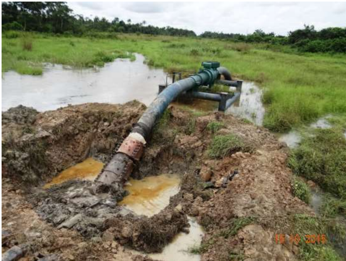
Overview: Part of spill impact on 20" KoloCreek – Rumuekpe Pipeline Right of Way at Aminigboko. Picture was taken during Joint Investigation of 15 th October 2015.
