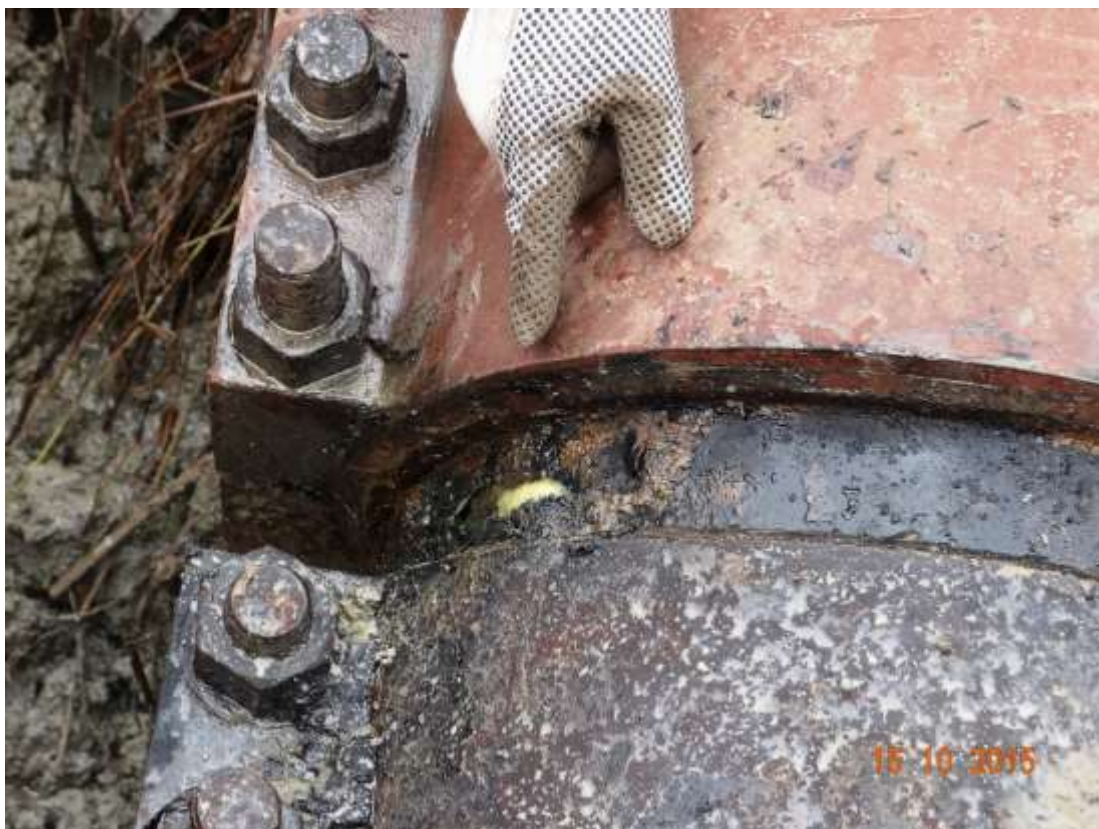
Close-up: Failed clamp on 20" KoloCreek – Rumuekpe Pipeline at Aminigboko. Picture was taken during Joint Investigation of 15 th October 2015.
