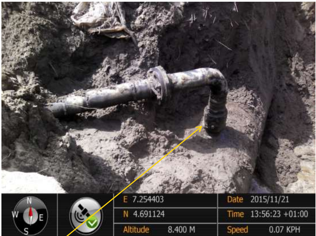
Close-up: Illegal fitting with concrete removed on 28" Nkpoku-Bomu Pipeline at B-Dere. Picture was taken during Joint Investigation of 21 st November 2015.
