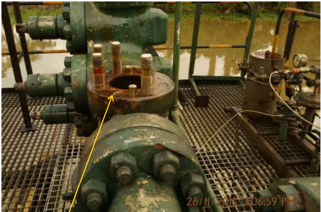
Close-up: Former position of Surface Safety Valve (SSV) on Benisede Well3T Wellhead at Ojobo. Picture was taken during Joint Investigation of 26 th November 2015.
