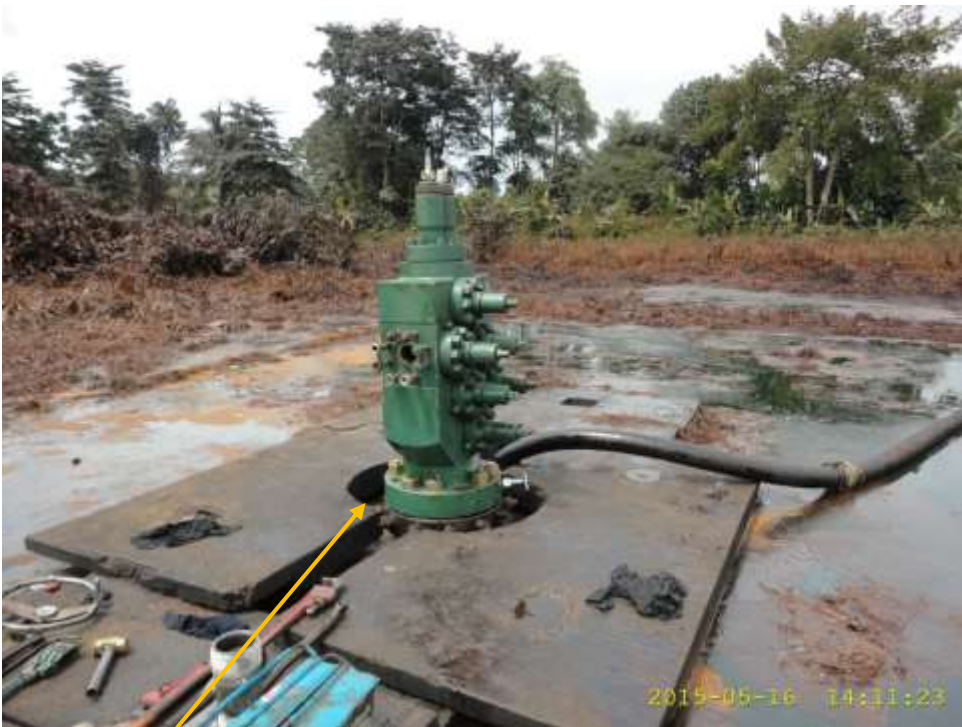
Close-up: Spill point after replacement of Nkali Well 11 wellhead at Okoroagu. Picture was taken during Joint Investigation of 16 th May 2015.
