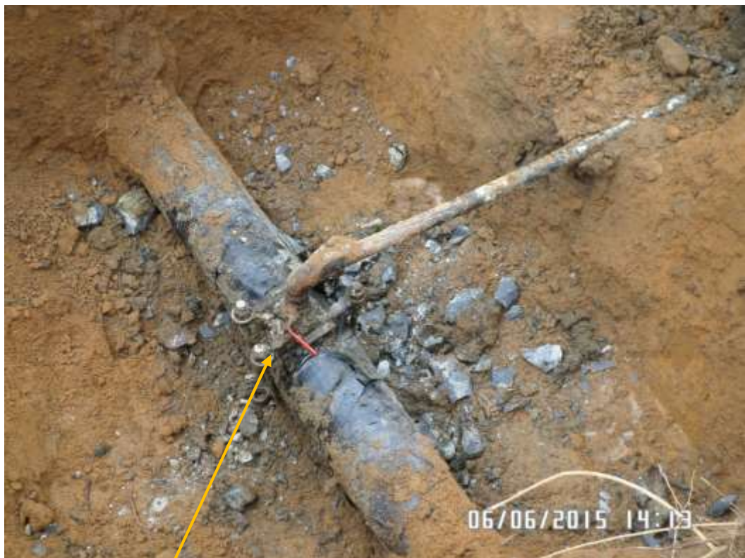
Close-up: Illegal fitting on 6" Obigbo – North Ogale Pipeline at Ogale. Picture was taken during Joint Investigation of 6 th June 2015.
