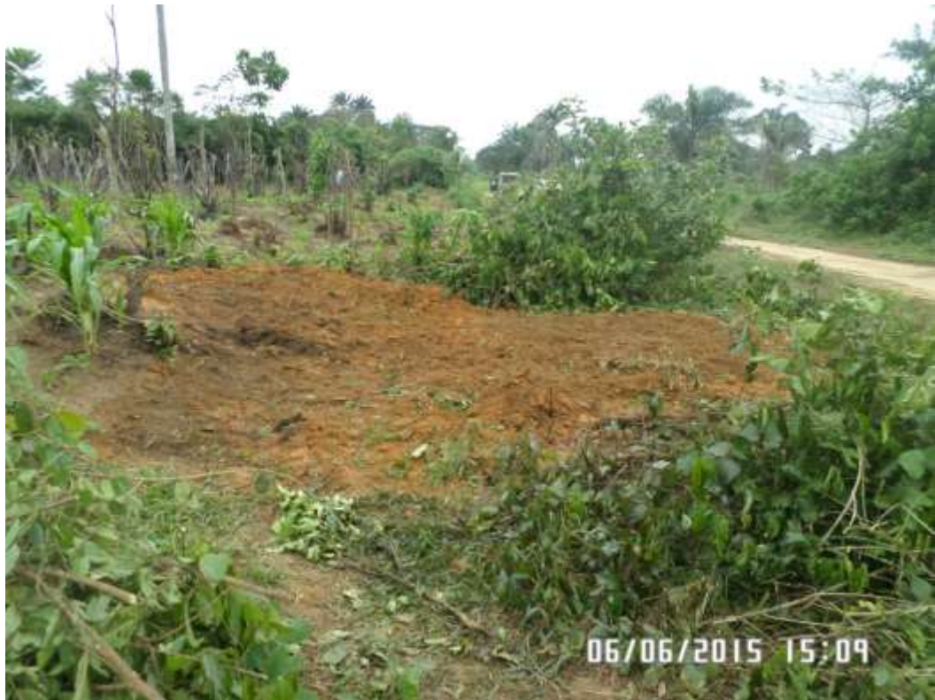
Overview: Part of spill impact on 6" Obigbo – North Ogale Pipeline Right of Way at Ogale. Picture was taken during Joint Investigation of 6 th June 2015.
