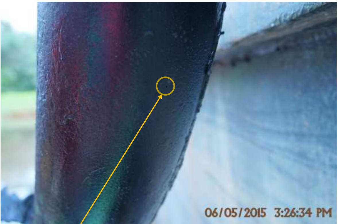
Close-up: Pinhole leak on Opukushi Well34T Flowline Riser at Agbidiama/Egbemo-Angalabiri. Picture was taken during Joint Investigation of 6 th May 2015.
