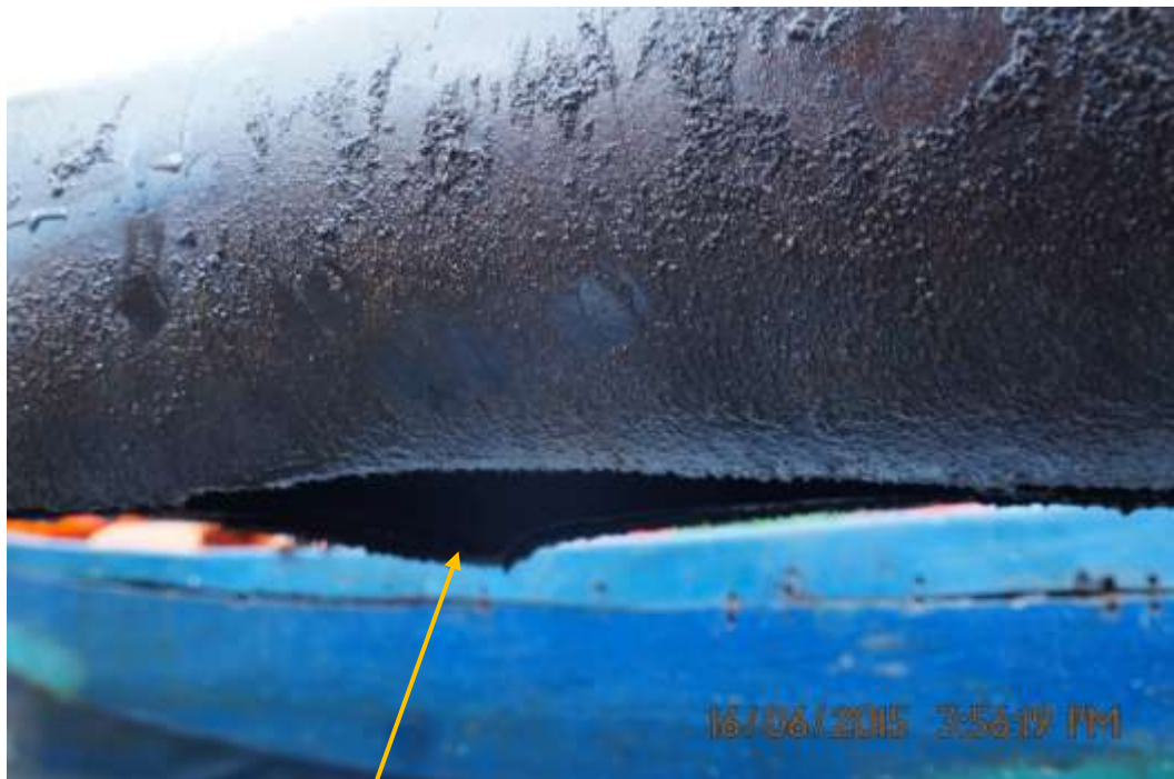
Close-up: Tear on Tunu Well6T Flowline at Agbidiana. Picture was taken during Joint Investigation of 16 th June 2015.
