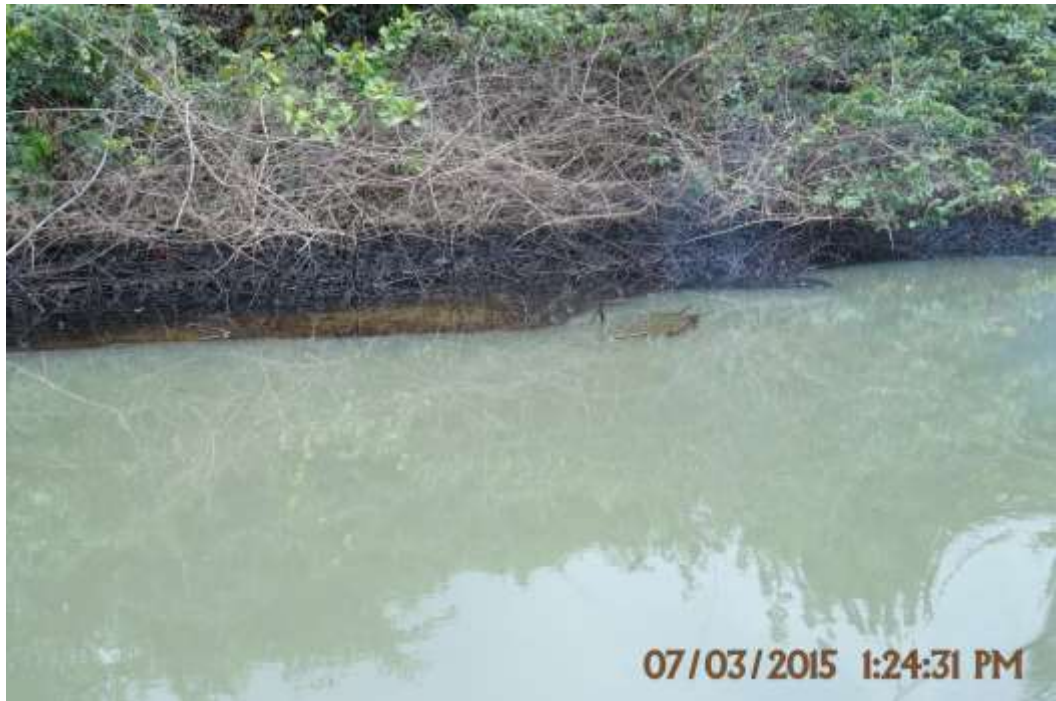
Overview: Part of spill impact on Tunu Well6T Flowline Right of Way at Agbidiana. Picture was taken during Joint Investigation of 7 th March 2015.
