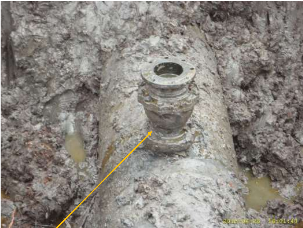
Close-up: Illegal fitting on 28" Bomu-Bony Trans Niger Pipeline at Bodo West. Picture was taken during Joint Investigation of 26 th April 2015.
