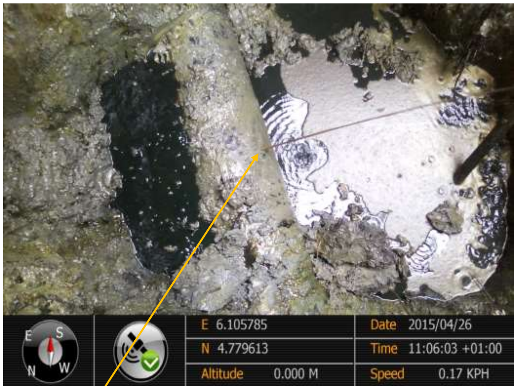
Close-up: Hacksaw Cut on 10" Diebu Creek – Nun River Pipeline at Oporoma. Picture was taken during Joint Investigation of 26 th of April 2015.
