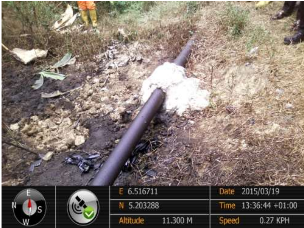
Overview: Part of spill impact on Adibawa Well10S Flowline Right of Way at Edagberi/Betterland. Picture was taken during Joint Investigation of 19 th of March 2015.
