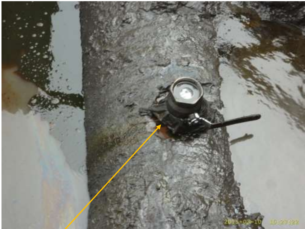
Close-up: Illegal fitting on 28" Bomu-Bonny Pipeline at BodoWest. Picture was taken during Joint Investigation of 10 th of March 2015.
