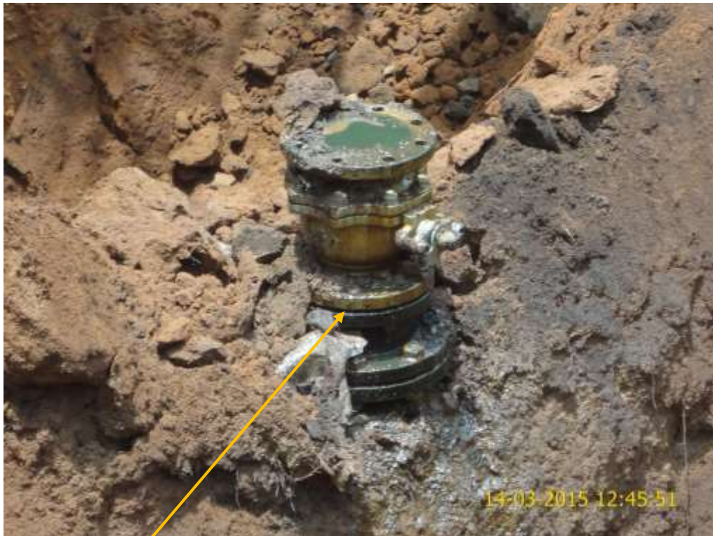
Close-up: Illegal fitting on 18" Assa-Rumuekpe Trans Niger Pipeline at Egbeda. Picture was taken during Joint Investigation of 14 th of March 2015.
