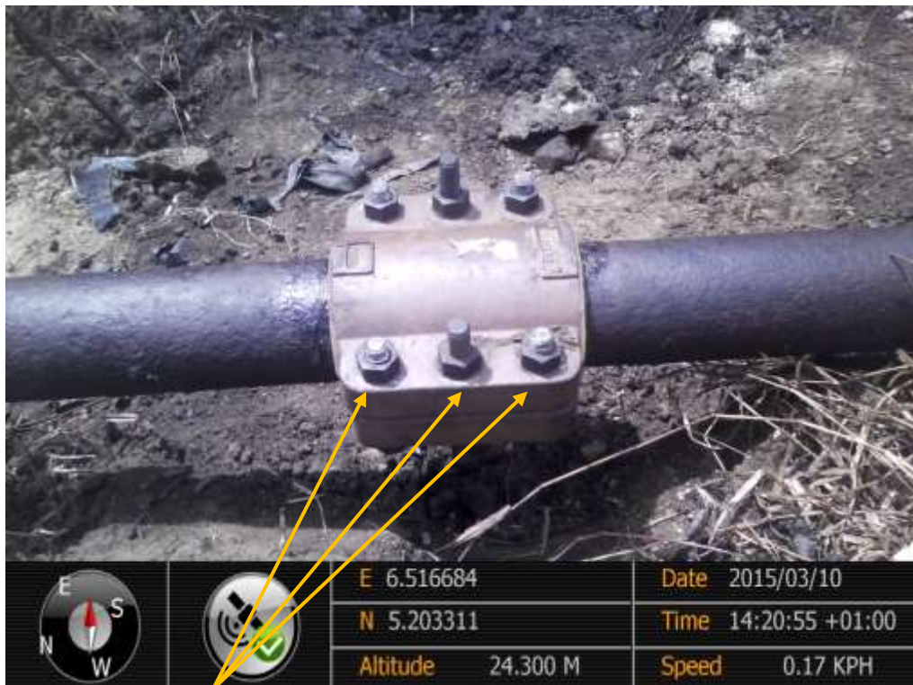
Close-up: Tampered nuts on Adibawa Well10S Flowline at Edagberi/Betterland. Picture was taken during Joint Investigation of 10 th March 2015.
