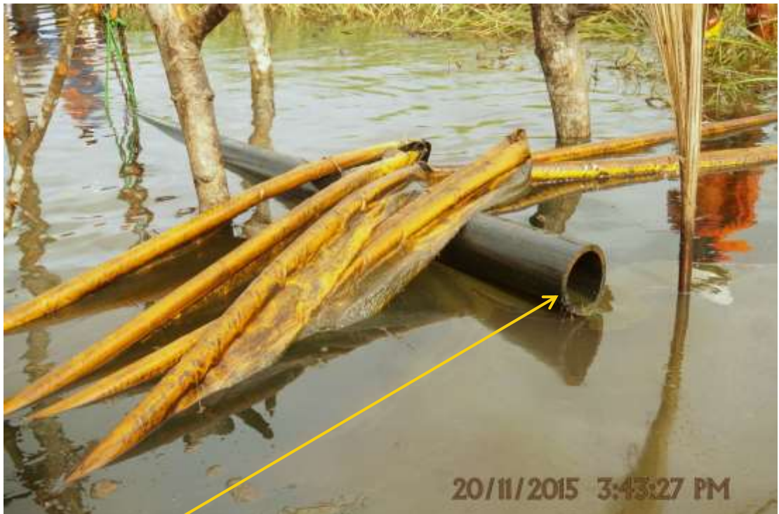
Close-up: Cut section of flowline on 6" Tunu – Kanbo Well4L Flowline at Agbidiama. Picture was taken during Joint Investigation of 20 th November 2015.
