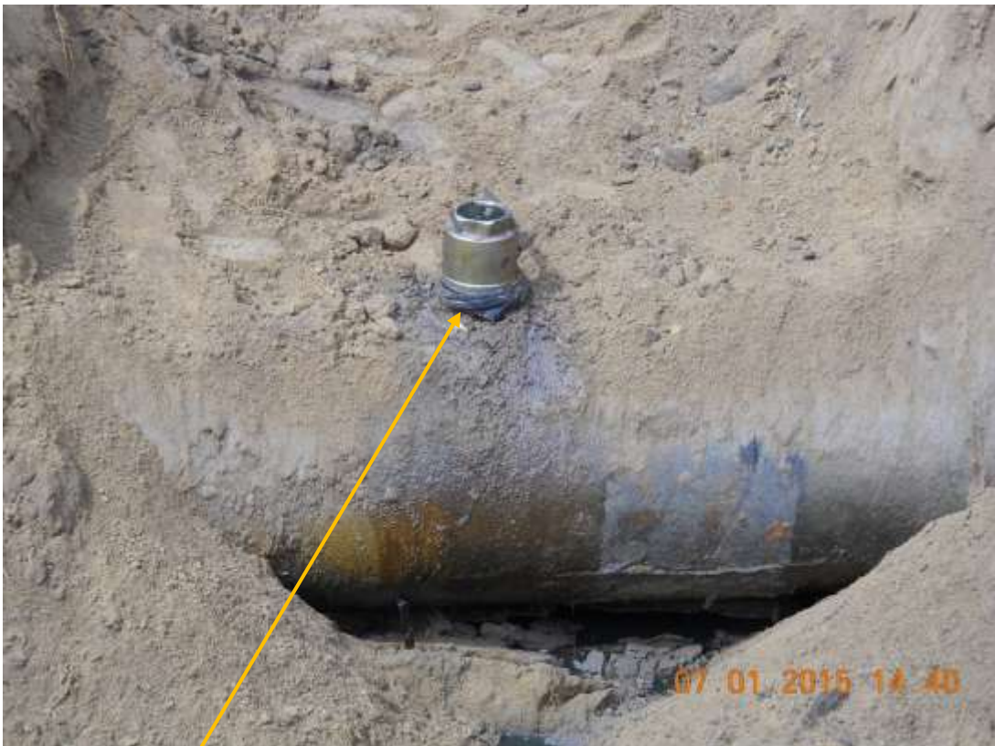
Close-up: Illegal fitting on 28" Nkpoku – Bomu Pipeline at B-Dere. Picture was taken during Joint Investigation of 1 st July 2015.
