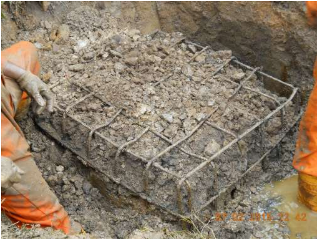
Close-up: Concrete cast found on 12" Imo River – Ogale Pipeline at Uzuaku. Picture was taken during Joint Investigation of 2 nd July 2015.
