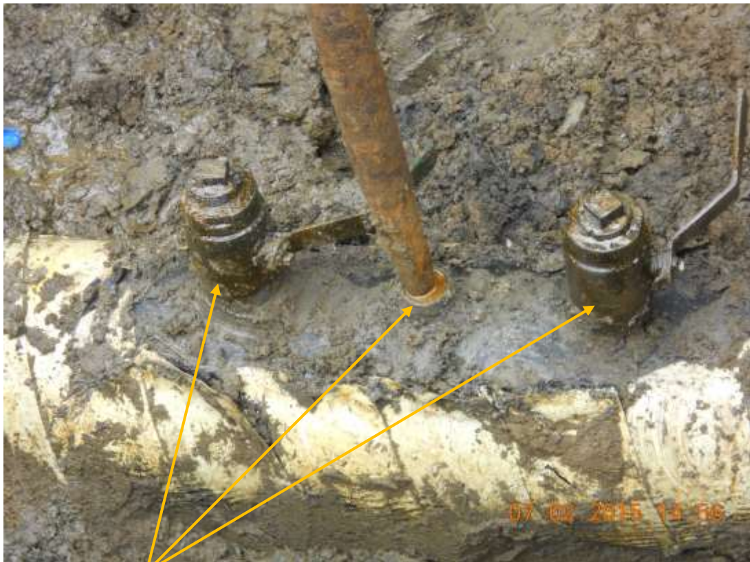
Close-up: Illegal fittings on 12" Imo River – Ogale Pipeline at Uzuaku. Picture was taken during Joint Investigation of 2 nd July 2015.
