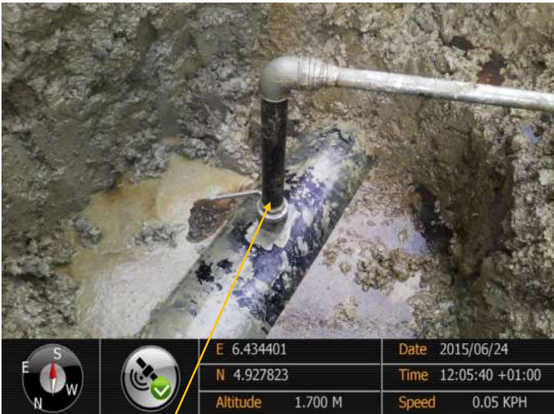
Close-up: Illegal fitting on 20" KoloCreek – Rumuekpe Pipeline at Odau. Picture was taken during Joint Investigation of 24 th June 2015.
