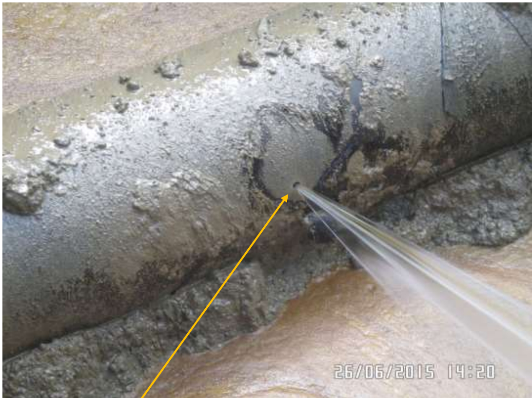
Close-up: Drilled hole on 18" Assa-Rumuekpe Pipeline at Elele/Alimini-Ihuaba. Picture was taken during Joint Investigation of 26 th June 2015.
