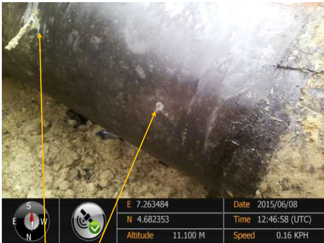
Close-up: Leaking and non-leaking drilled holes from previous incident on 28" Nkpoku-Bomu Pipeline at B-Dere. Picture was taken during Joint Investigation of 8 th June 2015.
