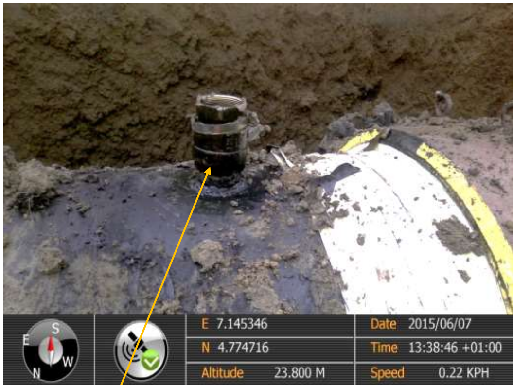
Close-up: Illegal fitting on 28" Nkpoku-Bomu Pipeline at Ejamah-Ebubu. Picture was taken during Joint Investigation of 7 th June 2015.
