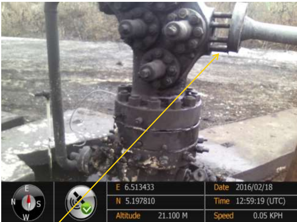
Close-up: Tampered Flange on Adibawa Well8SL Right of Way at Edagberi. Picture was taken during Joint Investigation of 13 th July 2015.
