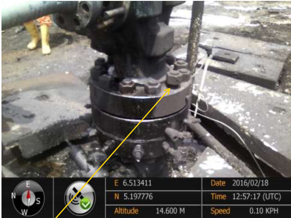
Close-up: Loosened bolts on Adibawa Well8SL at Edagberi. Picture was taken during Joint Investigation of 18 th February 2016.
