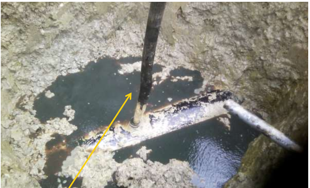
Close-up: Illegal fitting on 20" Kolo Creek to Rumuekpe Pipeline at Odau. Picture was taken during Joint Investigation of 28 th August 2015.
