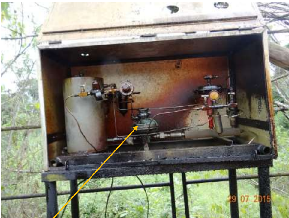
Close-up: Spill point on Adibawa Well 16T Wellhead at Edagberi. Picture was taken during Joint Investigation of 29 th July 2015.
