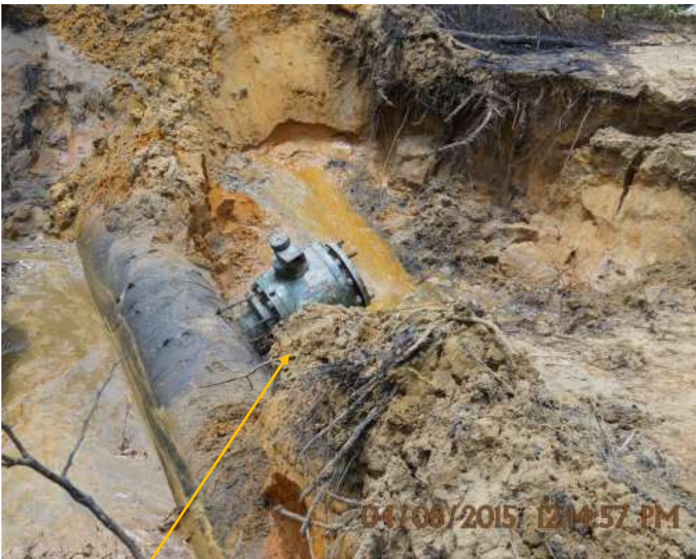
Close-up: Illegal fitting on 24" Trans-Escravos Pipeline at Burutu. Picture was taken during Joint Investigation of 4 th August 2015.
