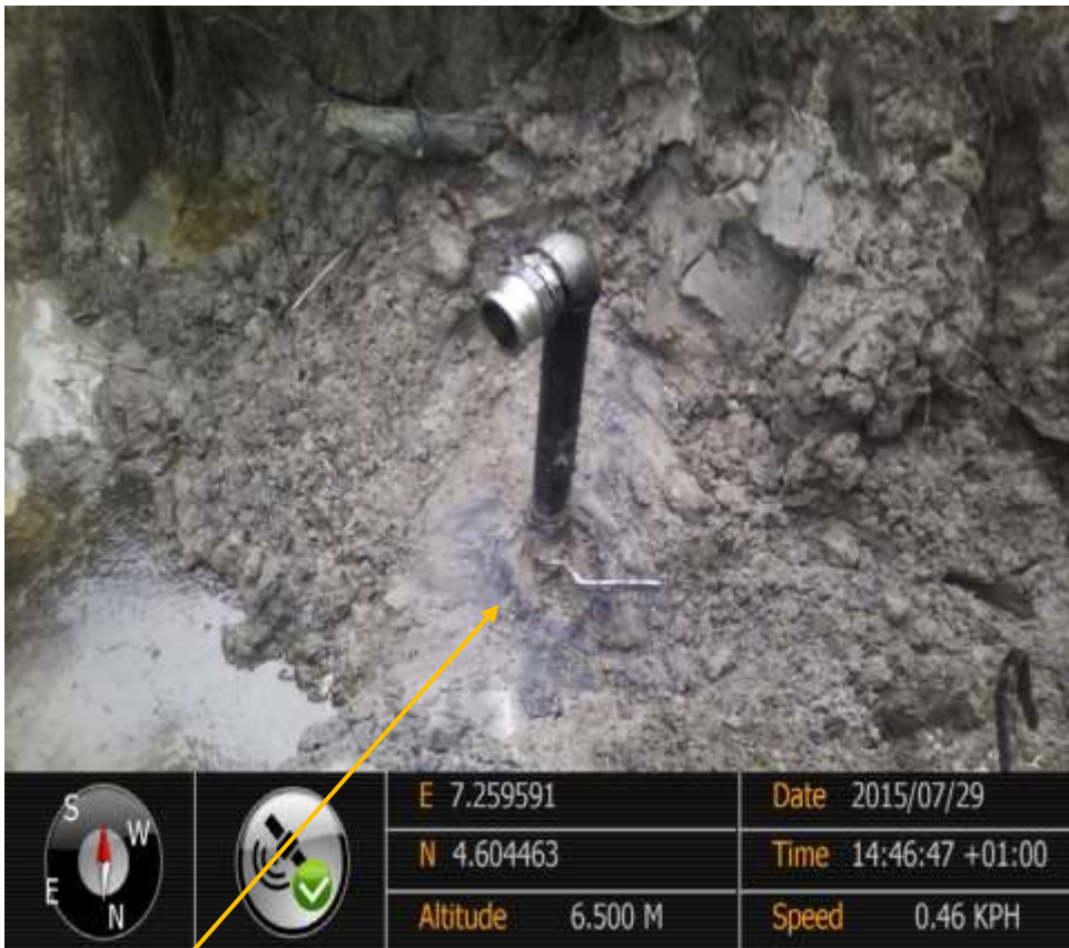
Close-up: Illegal fitting on 28" Bomu-Bonny Pipeline at Bodo-City. Picture was taken during Joint Investigation of 29 th July 2015.
