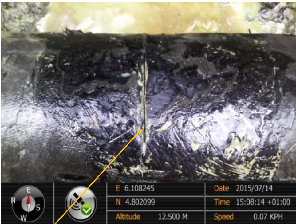
Close-up: Hacksaw cut on 10" Diebu Creek – Nun River Pipeline at Oporoma. Picture was taken during Joint Investigation of 14 th July 2015.
