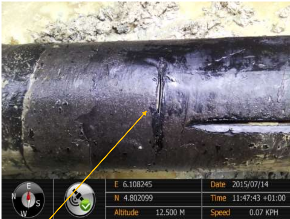
Overview: Hacksaw cut (B) on 10" Diebu Creek – Nun River Pipeline at Oporoma. Picture was taken during Joint Investigation of 14 th July 2015.
