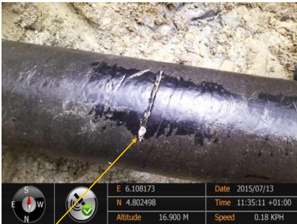
Close-up: Hacksaw cut (A) on 10" Diebu Creek – Nun River Pipeline at Oporoma. Picture was taken during Joint Investigation of 13 th July 2015.
