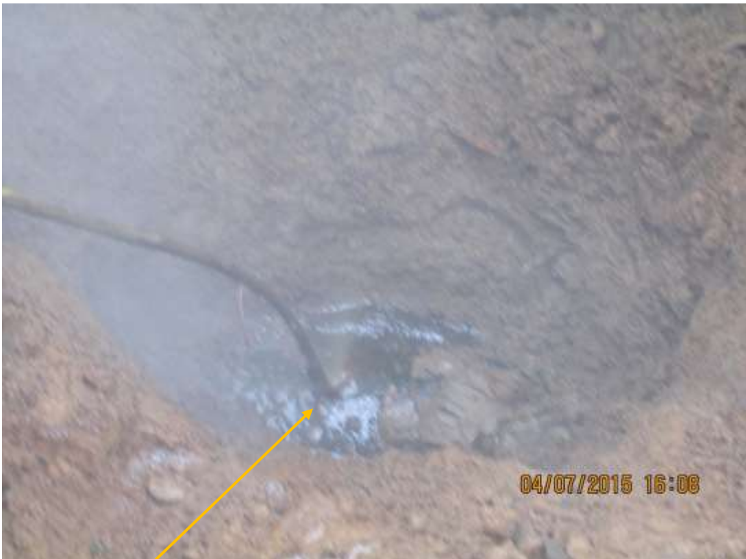
Close-up: Position of drilled hole pointed out by JIT member with stick on 8" Afam Well2 Flowline at Egberu. Hazing effecting picture clarity is due to gas leaking from drill hole.
