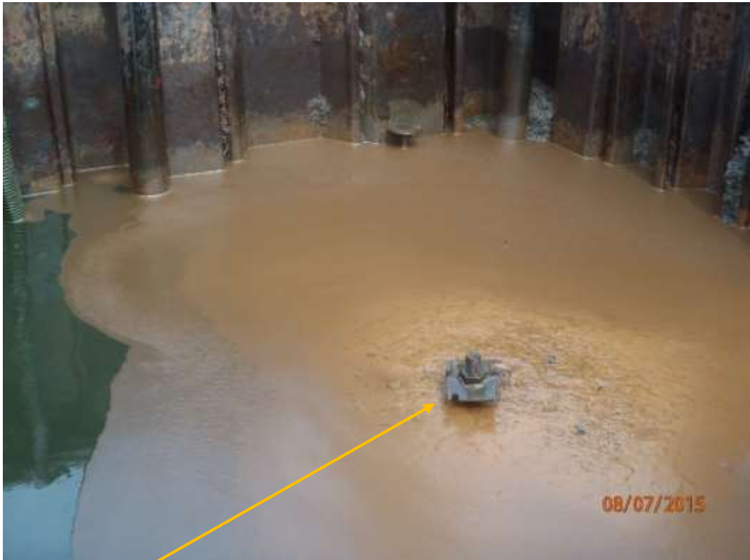
Close-up: Illegal fitting prior to temporary repair on 28" Bomu-Bonny Pipeline at Owokiri. Picture was taken during Joint Investigation of 8 th July 2015.
