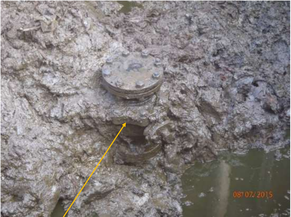
Close-up: Illegal fitting after temporary repair by blind flanging on 28" Bomu-Bonny Pipeline at Owokiri. Picture was taken during Joint Investigation of 8 th July 2015.
