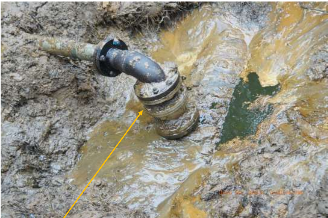
Close-up: Illegal fitting on 20" Otumara – Escravos Pipeline at Ogidigben. Picture was taken during Joint Investigation of 4 th July 2015.
