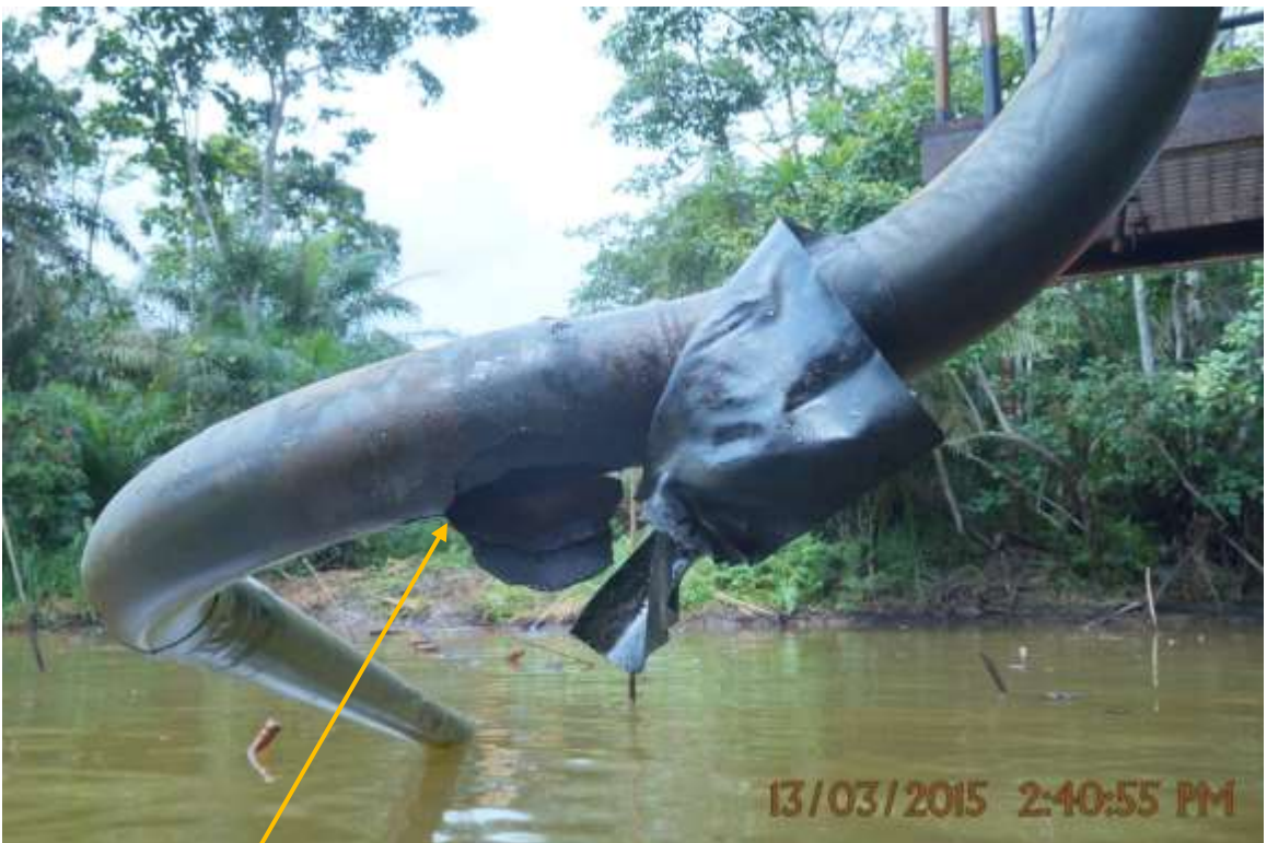
Close-up: Outward tear on Seibou Well2S Flowline at Gbanraun. Picture was taken during Joint Investigation of 13 th of March 2015.
