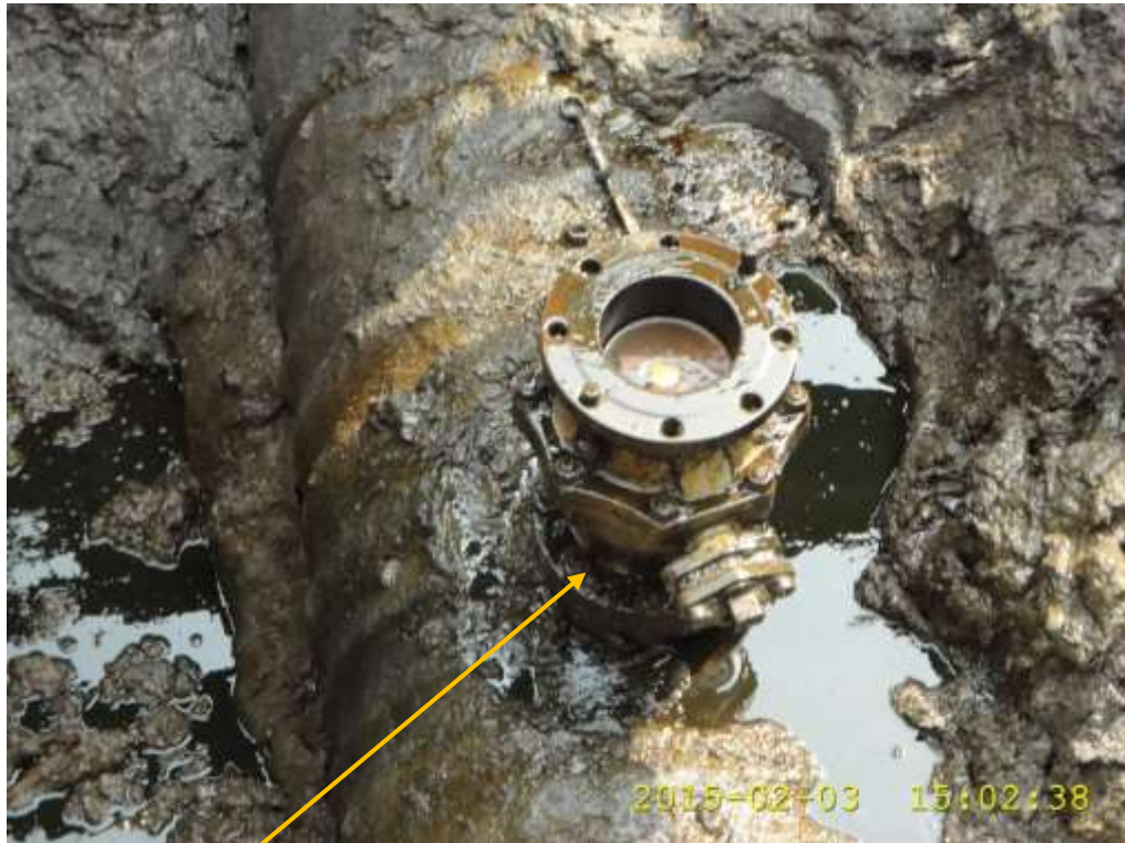
Close-up: Illegal fitting on 28" Bomu-Bonny Trans Niger Pipeline at Bodo West. Picture was taken during Joint Investigation of 3 rd February 2015.
