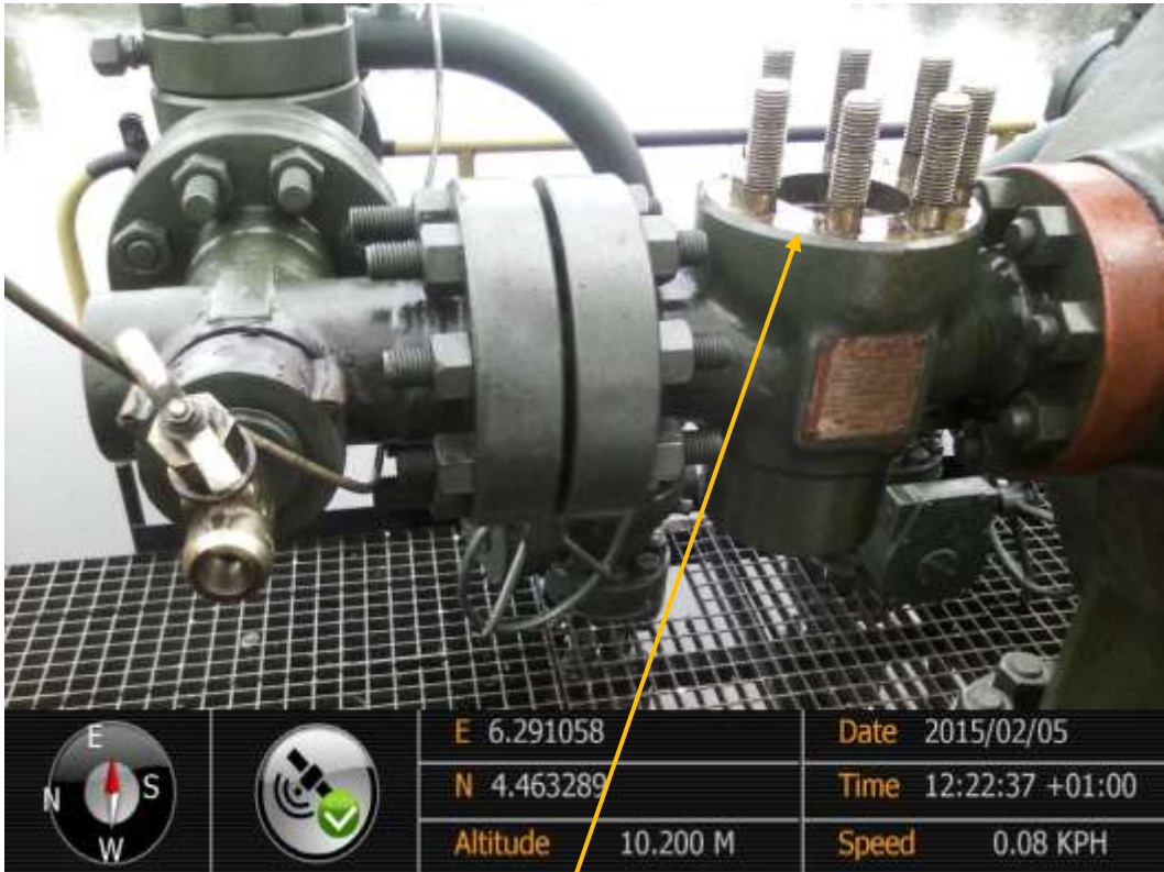
Close-up: Former position of missing Control Unit on Nembe Creek3 Well33S Wellhead at Ewelesuo. Picture was taken during Joint Investigation of 5 th February 2015.
