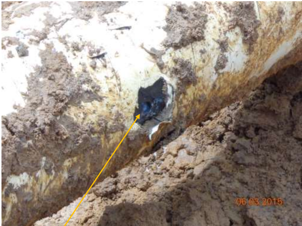
Close-up: Drilled hole on 8" Assa-Rumuekpe Pipeline at Imogu. Picture was taken during Joint Investigation of 6 th of March 2015.
