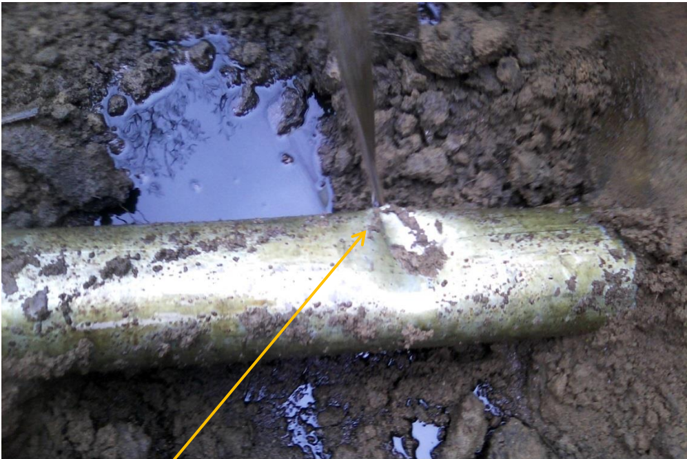
Illegal fitting on 28" Nkpoku - Bomu Pipeline at B-Dere. Picture was taken during Joint Investigation of 25th February 2015.
