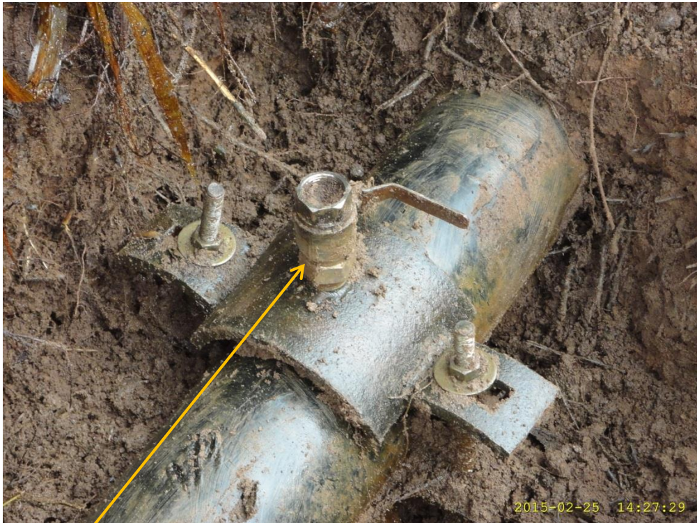
Close-up: Illegal fitting on Imo River Well 59T Flowline at Igirukwu. Picture was taken during Joint Investigation of 25th February 2015.
