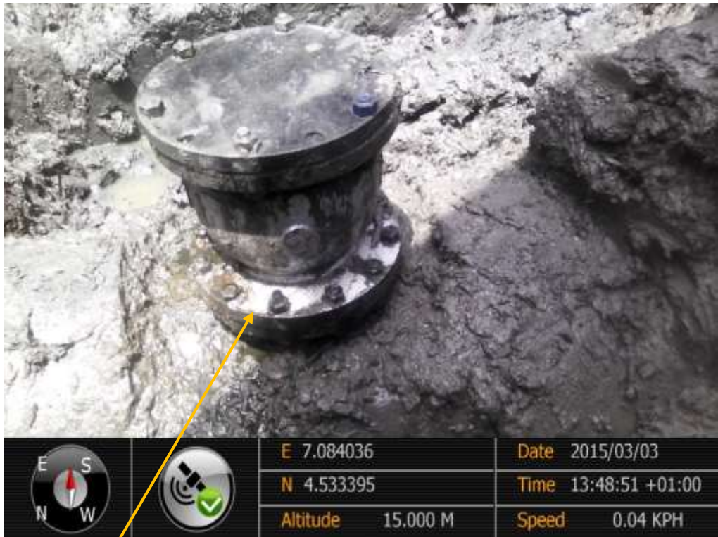
Close-up: Illegal fitting on 24" Nembe Creek Pipeline at Adamakiri. Picture was taken during Joint Investigation of 3 rd of March 2015.
